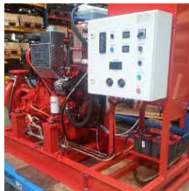
Customised Emergency Fire System
