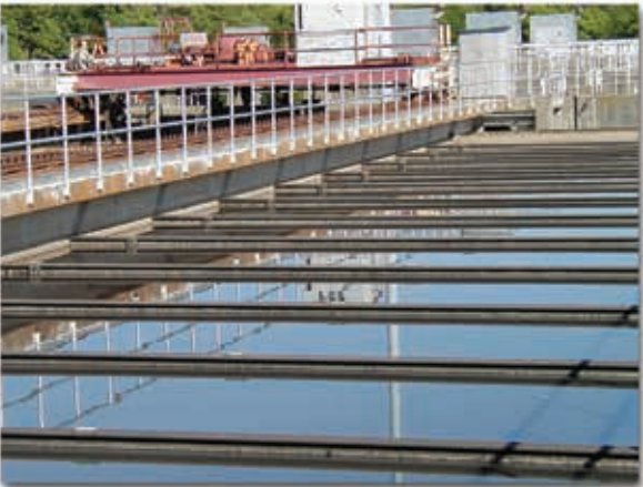
Closer view - 36 ft wide Clarifier with SAV 709 Chain
