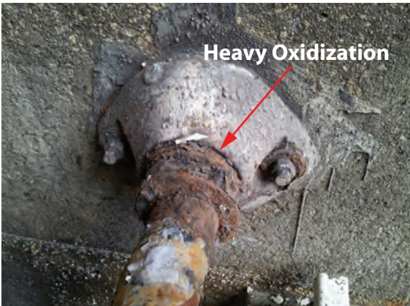
Metal Wall Bearing, corroded to the point that the shaft is frozen.
